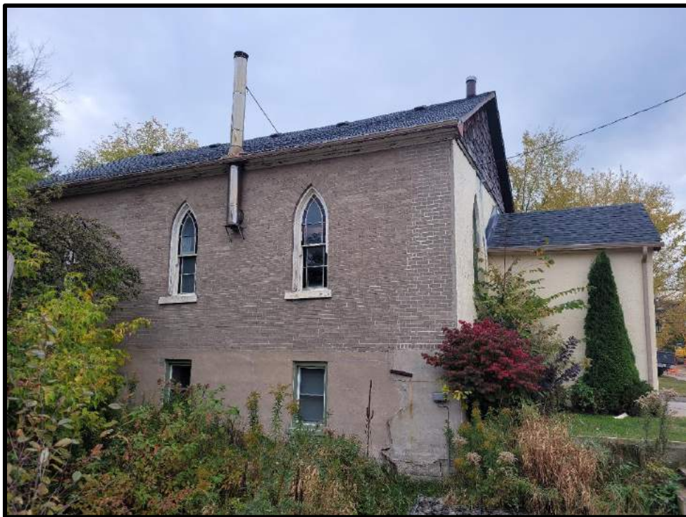
Image 6: North Elevation with Front Entrance of 93 Trafalgar Road (Photo taken on October 19, 2023; Facing East)
