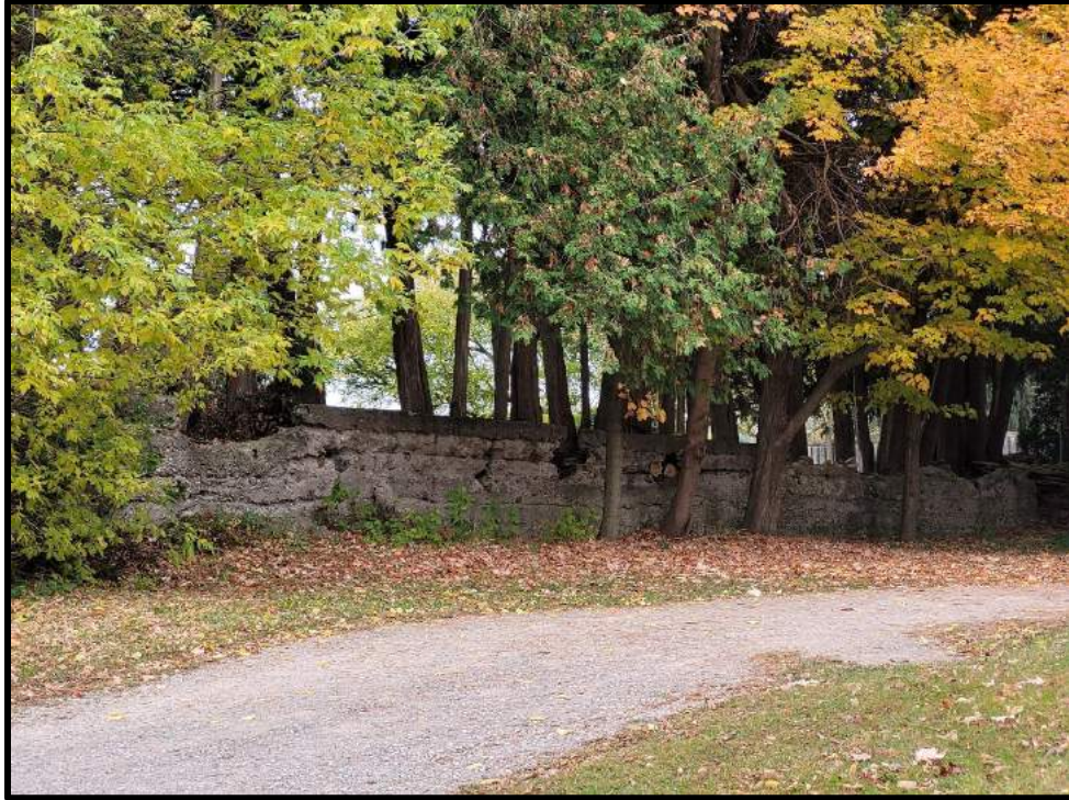
Image 9: Detailed View of Retaining Wall of 3 Station Street (Photo taken on October 19, 2023; Facing West)
