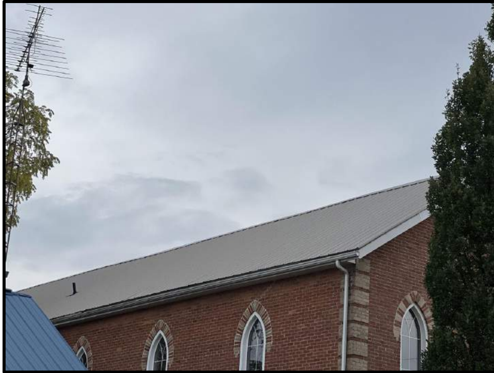
Image 11: Detail of Steel Roof of 21 Trafalgar Road (Photo taken on October 19, 2023; Facing Southeast)
