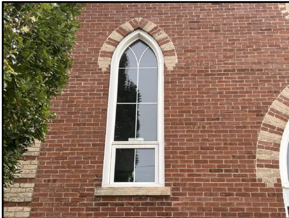
Image 4: Detail of Lancet Window Opening of 21 Trafalgar Road on Original Portion (Photo taken October 19, 2023; Facing Northeast)
