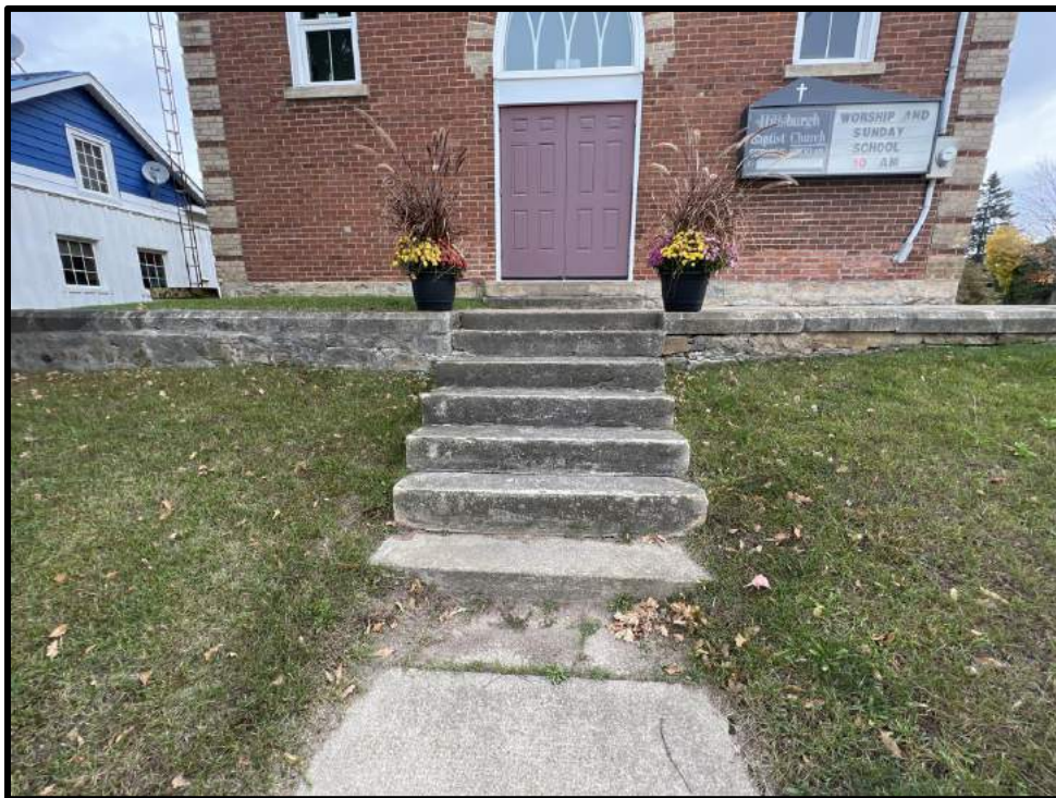
Image 6: Detail of Front Steps and Retaining Wall of 21 Trafalgar Road (Photo taken on October 19, 2023; Facing Northeast)
