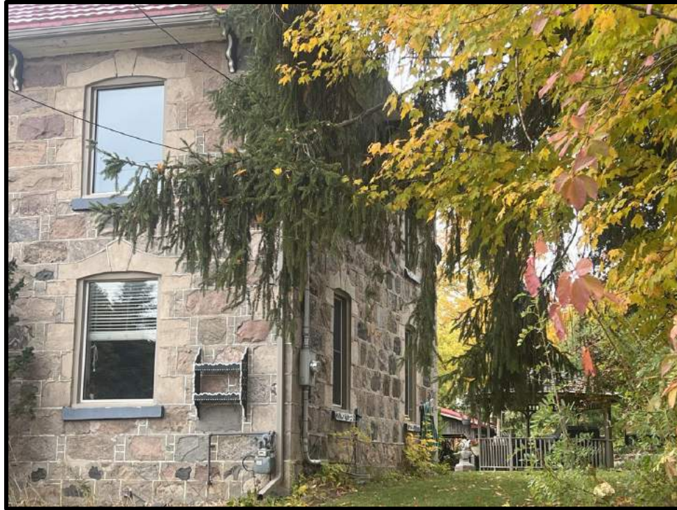
Image 3: Window Detail and North Elevation of 18 Anne Street (Photo taken October 19, 2023; Facing Southwest)
