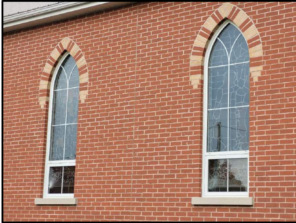
Image 5: Detail of Stain Glass Windows of 21 Trafalgar Road on Newer Portion (Photo taken on October 19, 2023; Facing Northeast)
